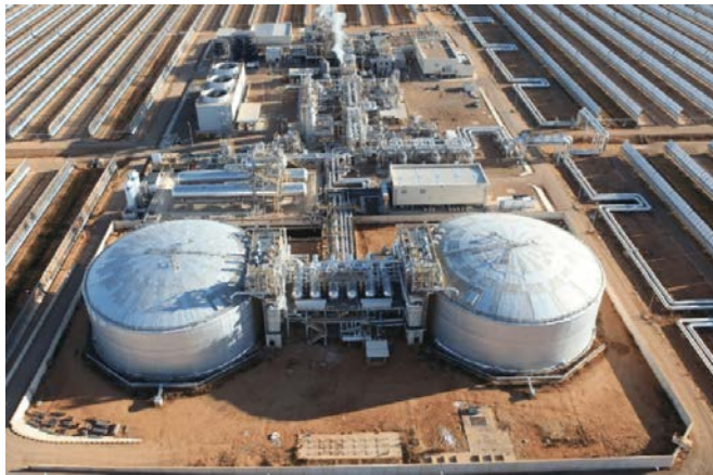
Figure 2 – Thermal storage tanks in Termosol 1 CSP Plant of 50 MW in Badajoz, Spain [11]
